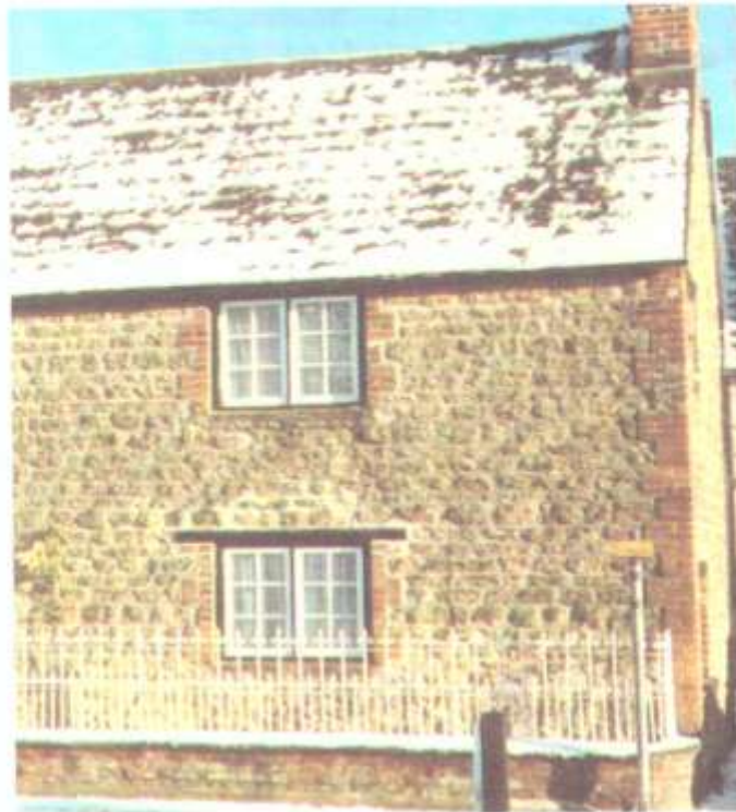
Fig.7. Part of the front face of a typical Faringdon house built in the mid 18th century. The facing stones are well and evenly dressed and well coursed. The lintels are of wood and bricks are restricted to the quoins, the chimney stacks and the door and window frames. The original tiles were probably Stonesfield slate.
